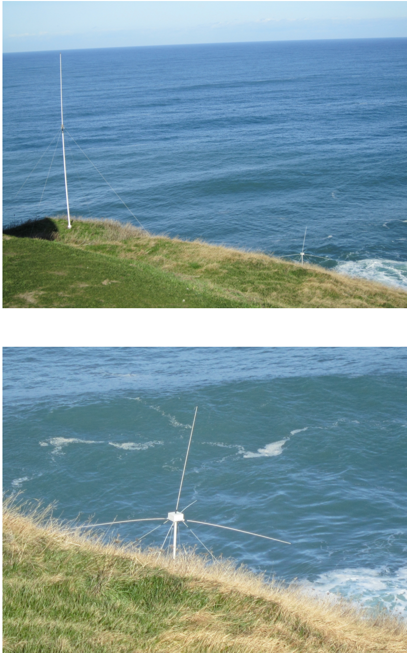
Figure 17: Matxitxako station antennae: (Up) transmitter antenna to the left and the receiver antenna to the right-down. (Down) receiver antenna (courtesy of Valentín Urgoiti).
