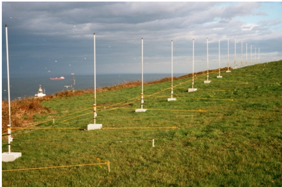
Figure 9: Example of WERA system's antenna installation (courtesy of T. Helzel)
