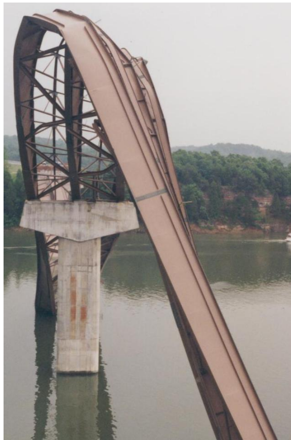
Figure 2. Collapse of State Route 69 Bridge over the Tennessee River at Clifton, Tennessee
