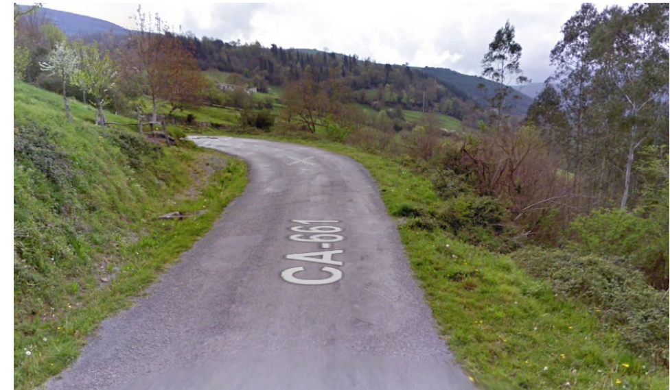
Figure 3: Absence of containment systems along the road.
