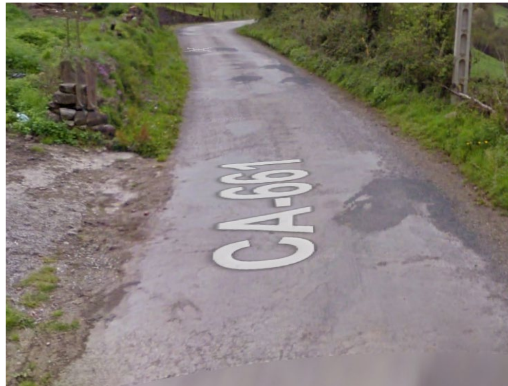
Figure 7: Road in poor condition and narrow for two-way traffic.
