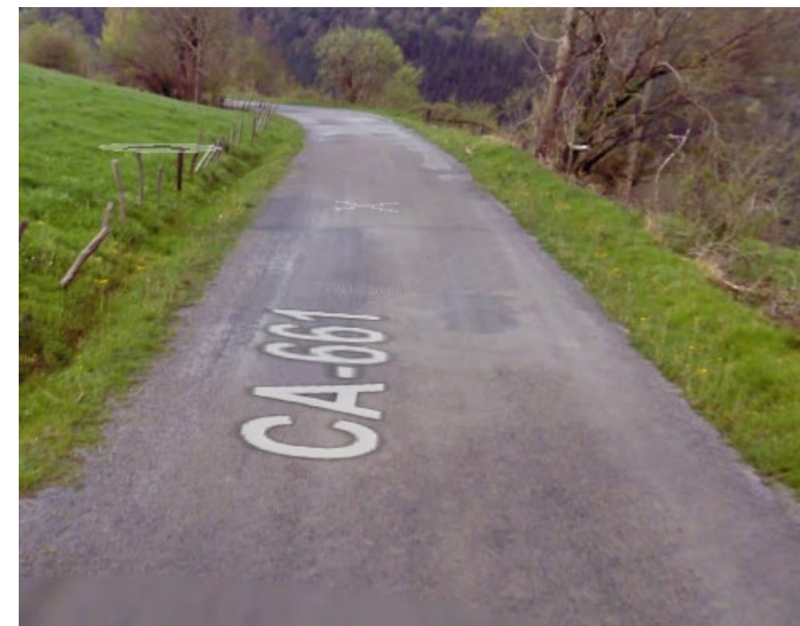
Figure 9: Absence of vertical signage along the entire route.
