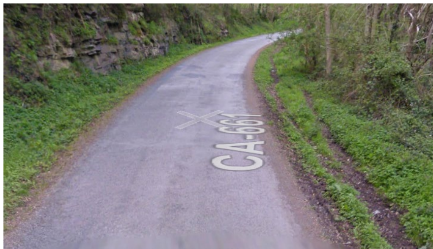
Figure 2: Absence of longitudinal drainage.
