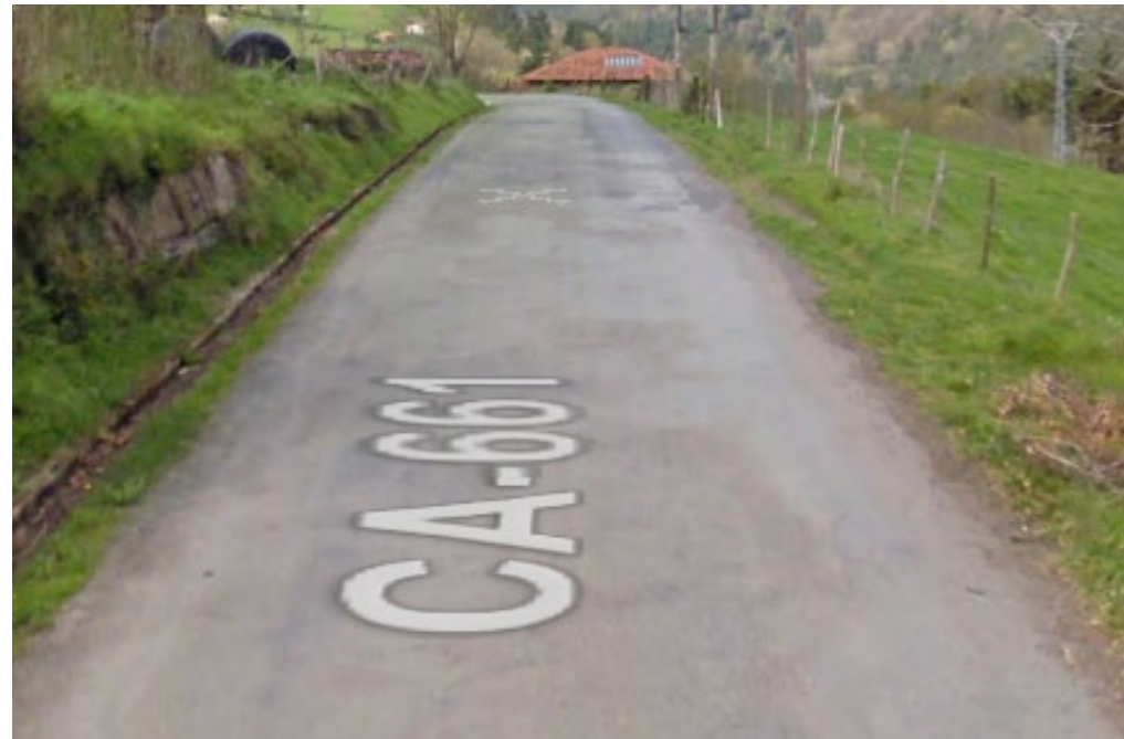
Figure 6: Absence of longitudinal road markings. No lane separation and no hard shoulders.
